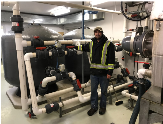
Neil Litchfield, CVRD Wastewater Treatment Plant
